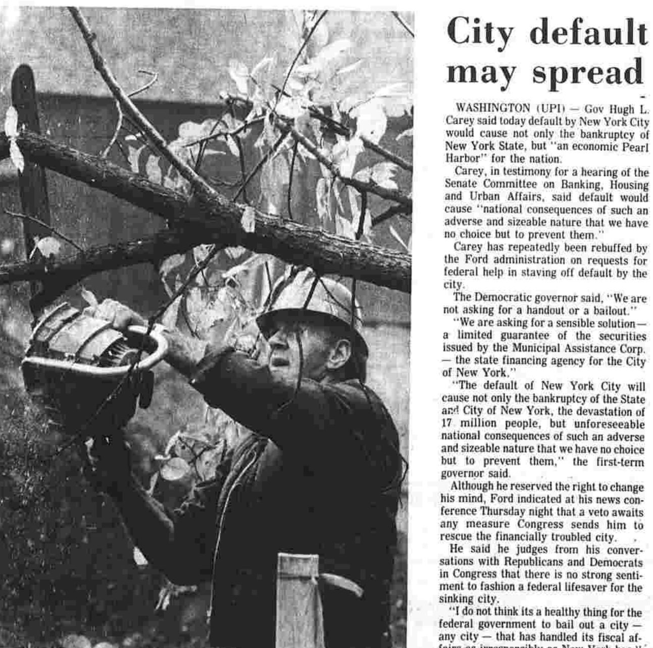
Clearing for firehouse Work on clearing the site for the Buckland Firehouse has started, following Wednesday's signing of a $233,000 contract for the project. Donald Beatty, an employee of Fred Brunoli & Sons of Avon, contractors for the construction, uses a chain saw to cut away shrubs and small branches. The firehouse will be at Tolland Pike, and N. Main St., adjacent and to the east of Buckland School. (Herald photo by Dunn)
